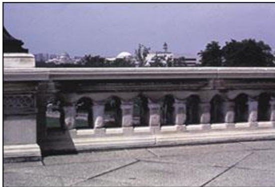
The marble balustrade on the west side of the Capitol building shows damage from acid rain dissolving the mineral calcite.
